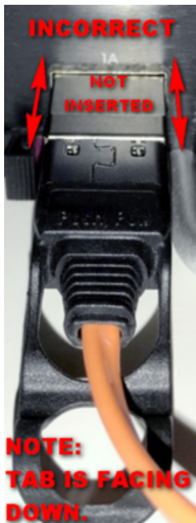
Figure 8. TippingPoint NX Series IPS – stacking port with the AOC cable installed incorrectly
